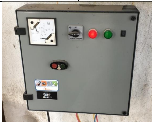
Switch to control the motor
